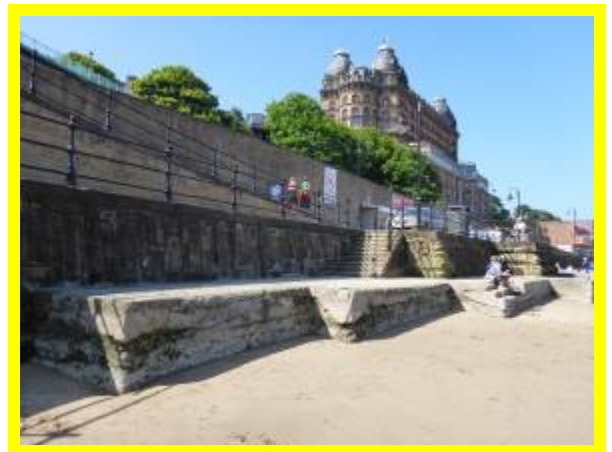
Abrasion of toe apron south of previous repairs (/1301C09)
