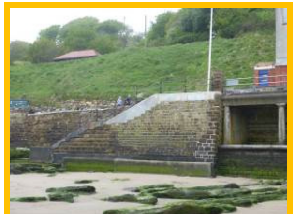
Previous repairs at southern tie-in following December 2013 storm damage (/1302C01)
