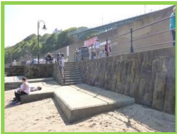
Previous repairs remain in good condition locally, but overall asset condition is fair (/1301C09)
