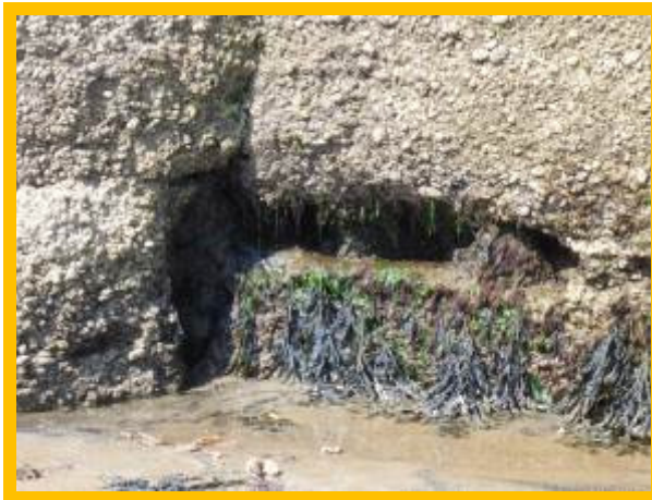
Void at toe in south face of West Pier wall (/1301C07)
