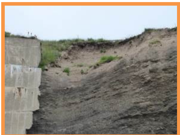
Erosion of cliffs immediately adjacent to large northern end of large sea wall (/1003C03)
