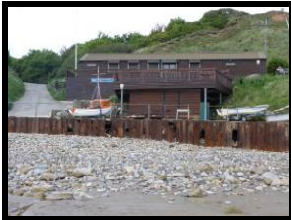
Failed central section of steel sheet piling as observed in May 2015 (/1601C01)
