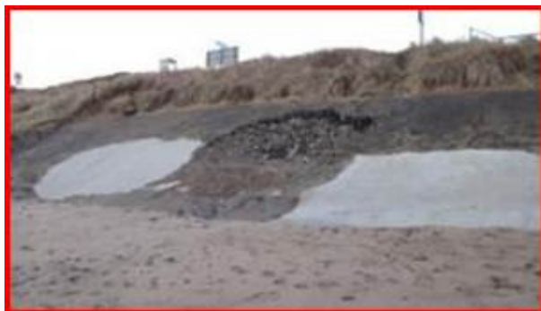
Previous storm damage and very poor condition of sloping revetment at Sandsend Road
