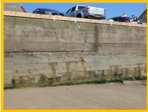
Longitudinal cold joints in south face of West Pier wall (/1301C07)
