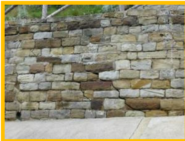
Diagonal cracking in stone wall (/0601C06)
