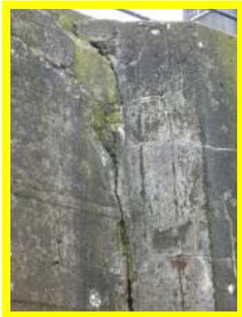
Full height vertical crack (/0403C01)
