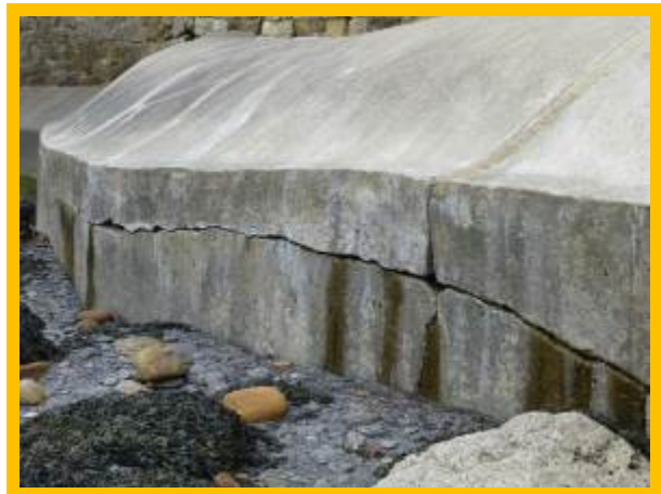
Longitudinal cracking in concrete toe apron (/0601C06)
