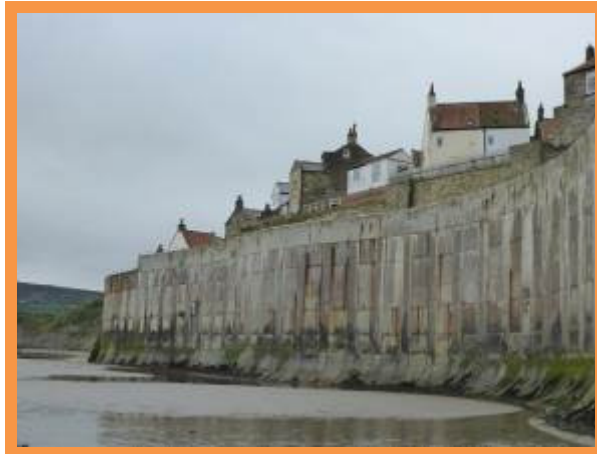
Large sea wall in poor condition will benefit from future planned capital scheme (/1003C02)
