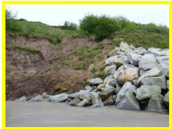
Slumping of cliffs immediately adjacent to southern end of rock armour (/1003C07)
