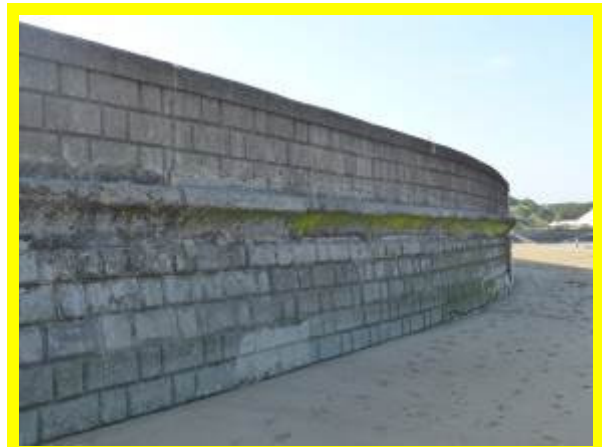
Area of heavy abrasion damage to promontory wall (/1201C04)
