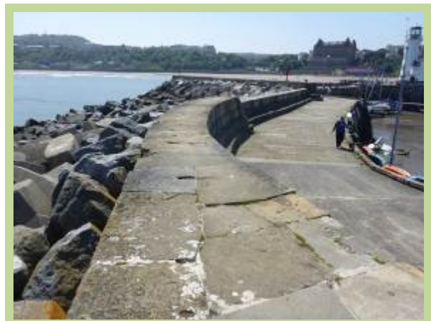
Abrasion towards seaward end of East harbour outer wall (/1301C01)
