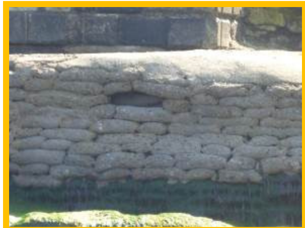
Gaps in need of filling (/1302C02)
