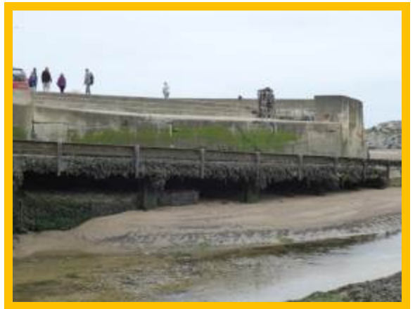
Cracks and cold joints in concrete seawall to rear of slipway (/0402C03)
