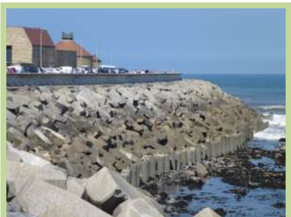
Accropode revetment with concrete toe piles, rock crest and wave return wall (/1202C04)
