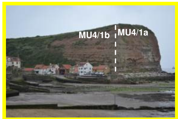
East-facing Cowbar Nab MU4/1a (right) (Partly Active in June 2016) and south-facing Cowbar Nab along Staithes Beck MU4/1b (left) (Locally Active in June 2016)
