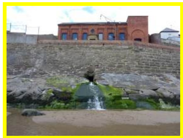
Private sea wall in fair overall condition but with the toe apron subject to ad hoc repairs (/1402C05)
