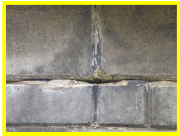
Occasional open joints with missing mortar (/1602C06)
