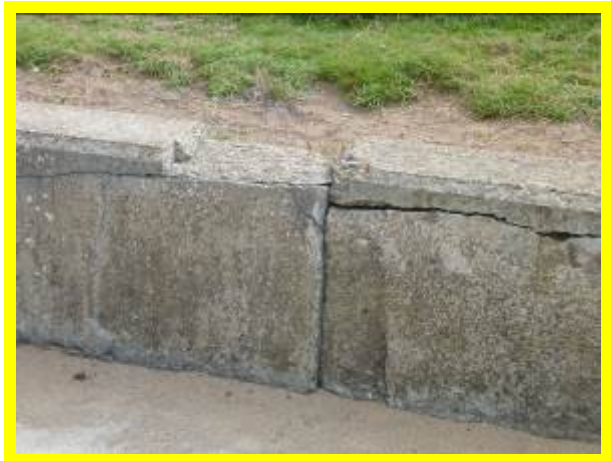
Damage to low wall at rear of promenade (D0801C01)
