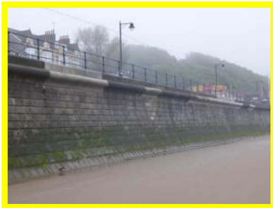
Previous repairs to coping and wave return feature (/1602C08)
