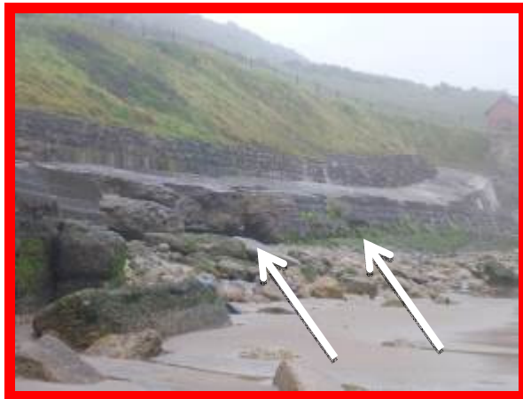
Sea wall in very poor condition with areas of significant undercutting and areas of missing blockwork leading to large voids (/1402C04)
