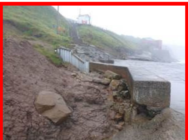
Slumping cliffs adjacent to steps leading to outflanking – southern end (/1402C04)
