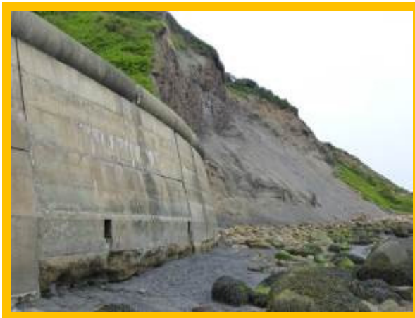
Sea wall with undermining, surface cracks and heavy abrasion – note erosion of undefended cliffs to north (/0601C01)
