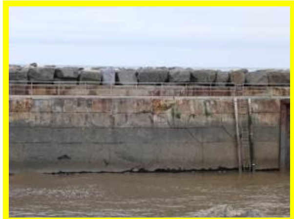
Undercutting to a significant length of the inner-facing wall of North Breakwater (/0402C01)
