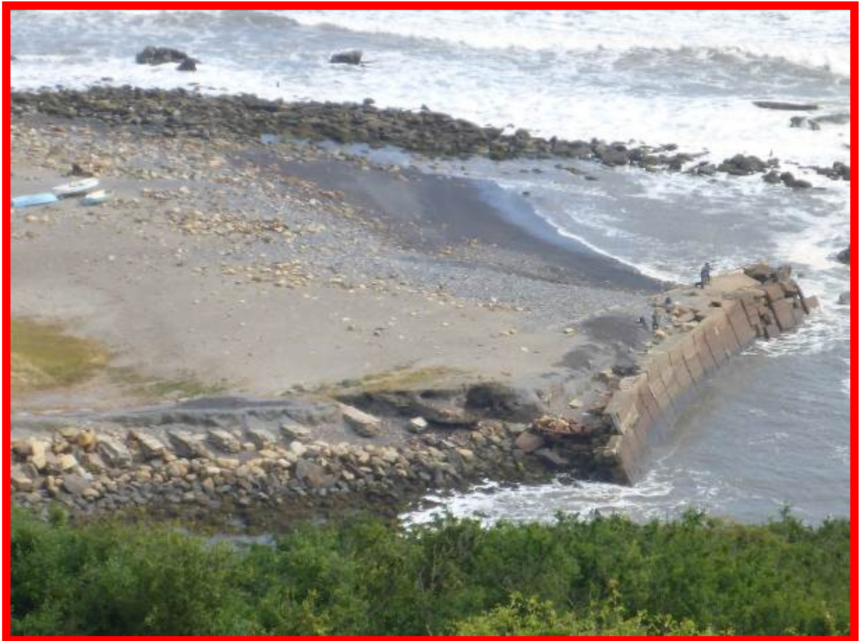
Dilapidated asset in 2016 (\D0502C01)
