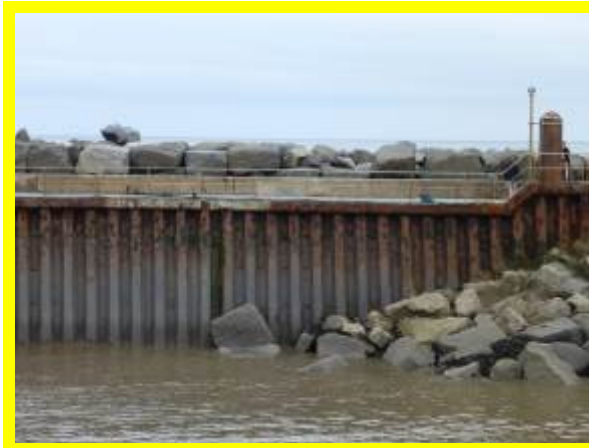
Corroded steel sheet piling on inner-face of North Breakwater (/0402C01)
