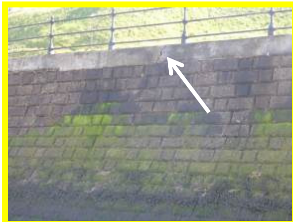
Small crack in coping of seawall (/1201C21)
