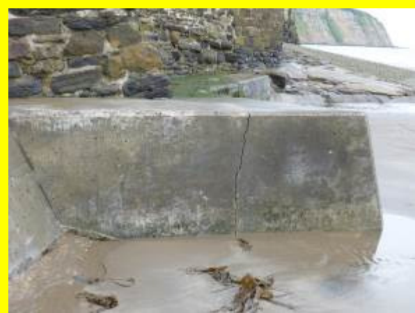
Typical defects (cracking) on toe apron (/1003C06)
