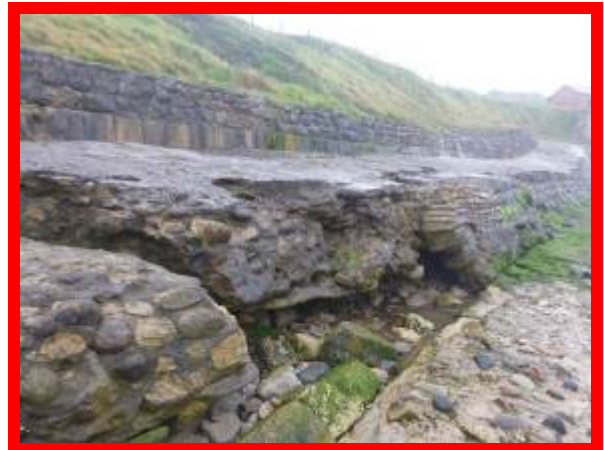
Undercutting at toe leading to voiding behind and break-up of deck (/1402C04)
