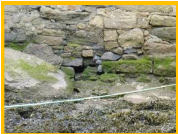
Wall on northern side of beck (missing blocks, open joints and voids) (/0402C06)
