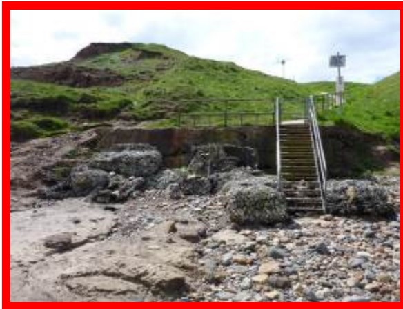
Failed gabion baskets at surf shop car park beach access (no asset reference)
