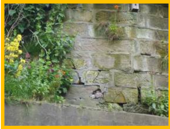
Cracking, open joints and vegetation growth (/0402C04)
