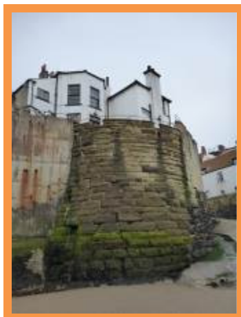
Blockwork wall in poor condition fronting the Bay Hotel (/1003C04)
