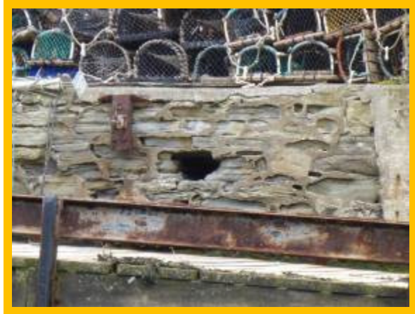
Missing blockwork in stone wall to rear of slipway (/0402C03)
