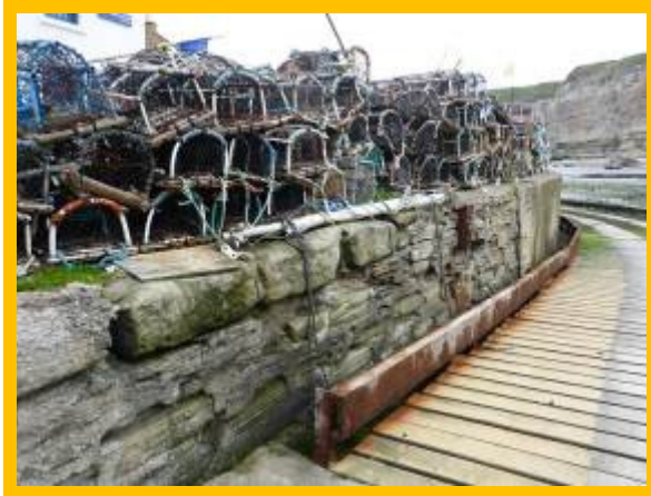
Poor condition stone wall to rear of slipway (/0402C03)
