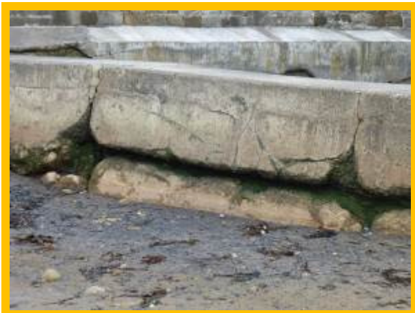
Previous repairs to toe apron next to heavily abraded section (/0601C02)
