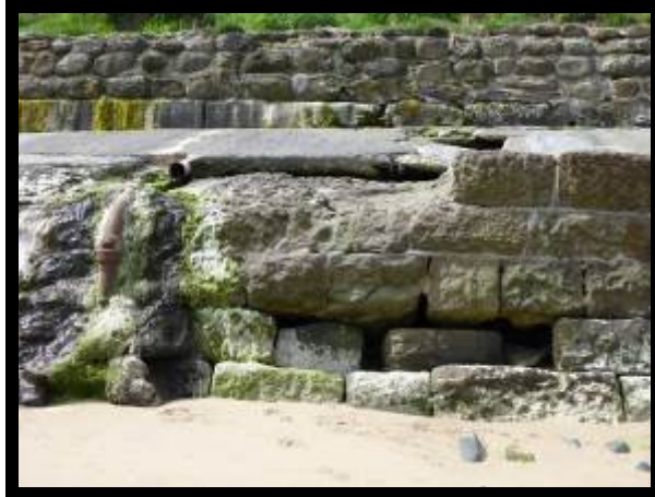
Missing blockwork in May 2015 (/1402C04)
