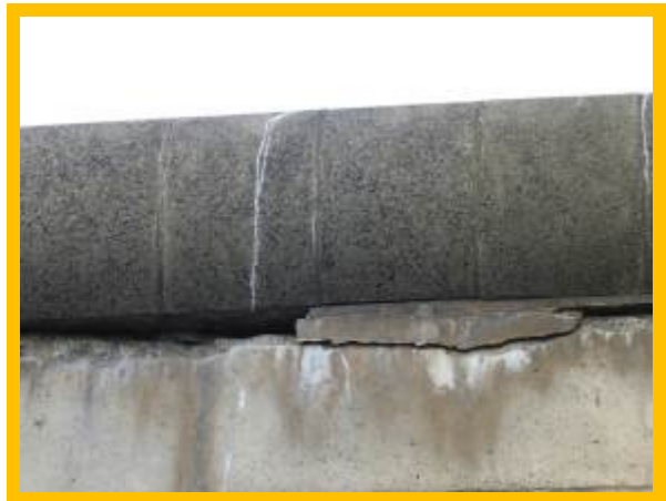
Wash out of joints under the capping beam (/0601C01)
