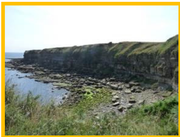
MU19/6 Rockfall on southern side of Cloughton Wyke (Partly Active)
