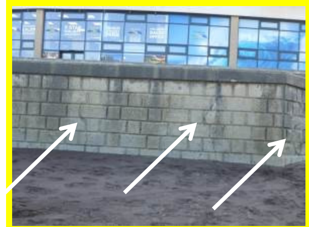
Vertical cracks in wall protecting recent development (/1201C06)
