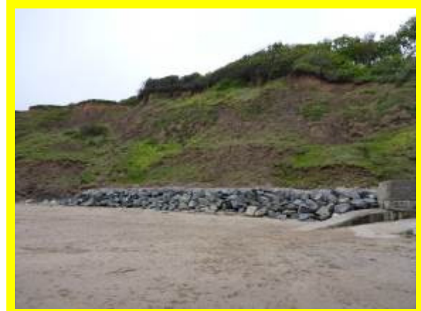
Rock revetment at southern end of Filey Sea Wall (/1602C02) – note active coastal slopes to rear
