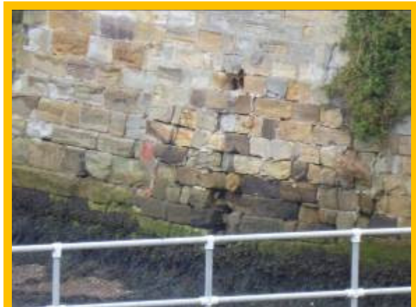
Local poor condition of quay wall due to open joints between blocks (\803C06)
