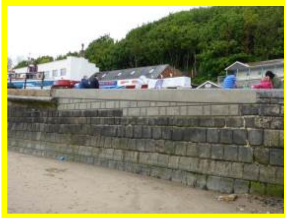
Previous repairs to slipway 'wing-wall' holding well (/1602C09)
