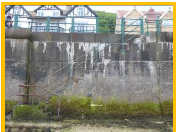
Particular defects at access steps (D0702C01)
