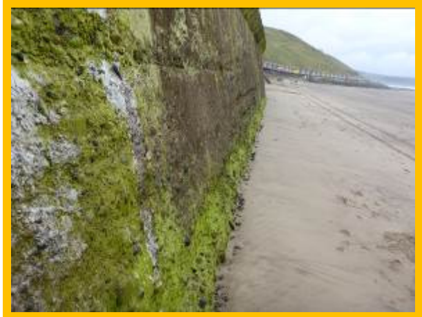
Abrasion damage to sea wall face (D0802C03)
