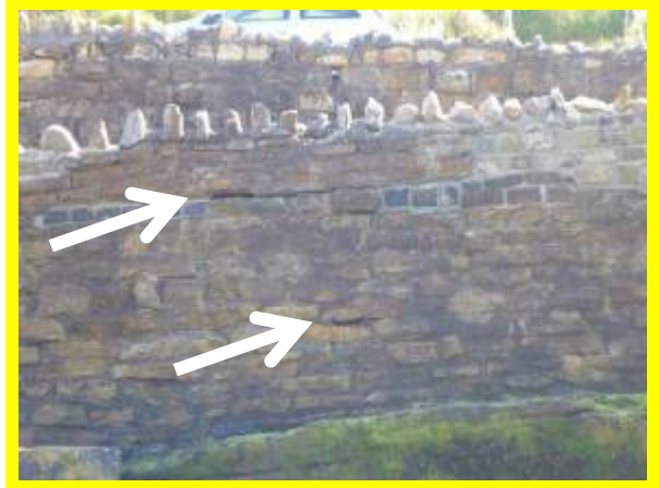
Gaps in need of filling (/1302C03)
