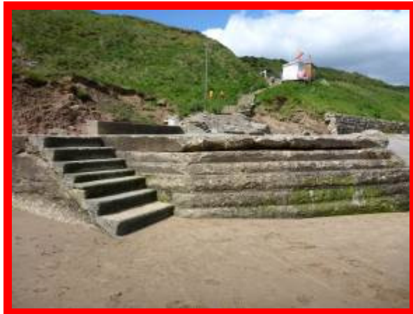
Landing at beach access and slumping cliffs adjacent to steps (/1402C06)
