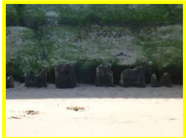
Exposed timber toe piles (/1301C26)
