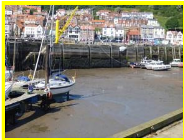
Wall of Vincent Pier facing East Harbour covered by timber boarding and algae (/1301C04)
