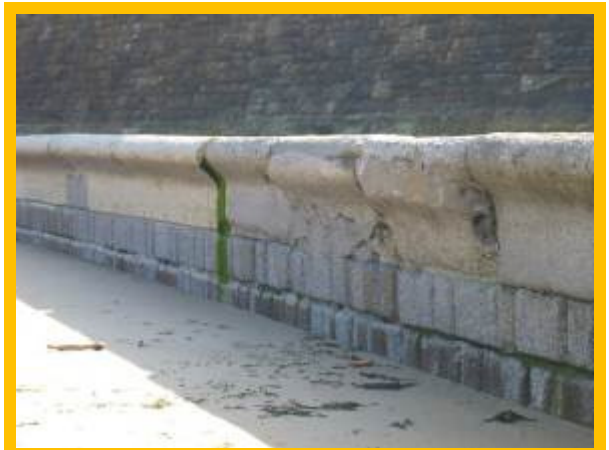
Seawall in overall fair condition although with heavy abrasion damage locally (/1304C02)
