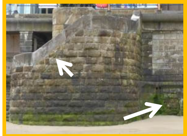
Crack in wall and displacement/loss of facing masonry in blocks at toe (/1301C29)
