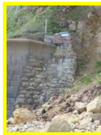
Erosion of undefended cliffs at tie-in of sea wall private sea wall (/1402C02)
