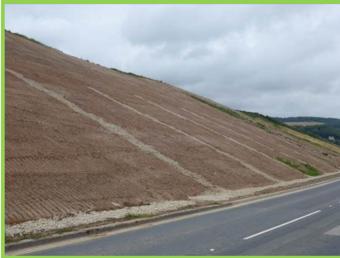
MU9/3 Coastal slopes to rear of new sea defences in an inactive state following capital works involving re-grading, drainage and seeding as part of the Sandsend Road Coast Protection & Slope Stabilisation Scheme
