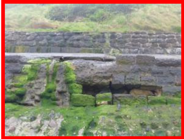
Further missing blockwork in June 2016 (/1402C04)
