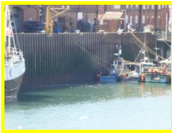
Corroded steel sheet piling on inner face of West Pier (/1301C13)
