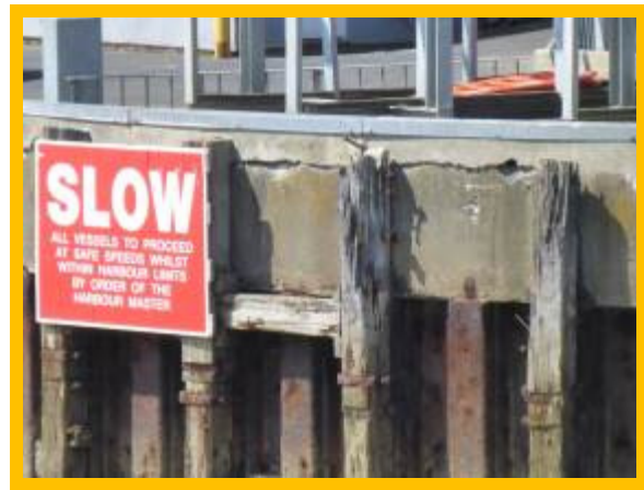
Corroded steel and cracked capping beam on seaward end of West Pier (/1301C1718)
