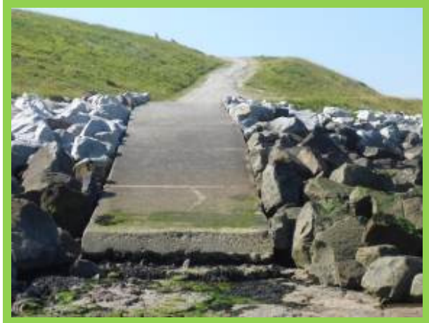
Vertical drop and crack in concrete at end of access ramp at south end of revetment (/1304C01)
