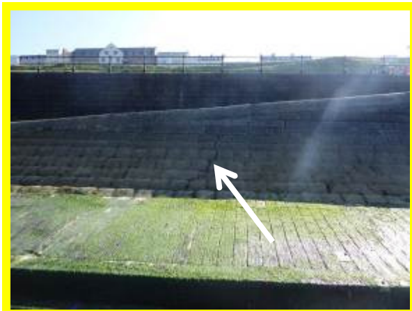
One of two notable cracks visible in wing-wall at access ramp (/1201C21)
