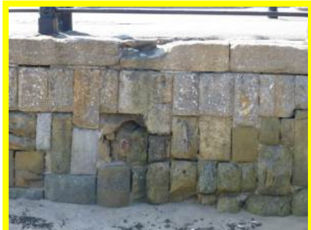
One of the worst areas of abrasion and open joints (/1301C25)
