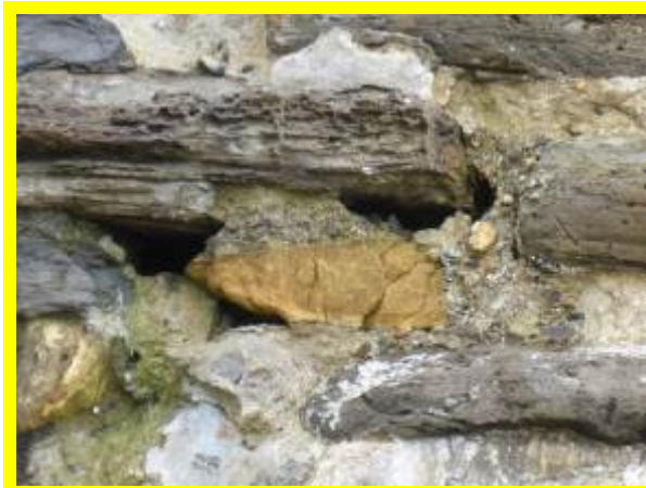
Typical defects (gaps) on blockwork wall (/1003C06)
