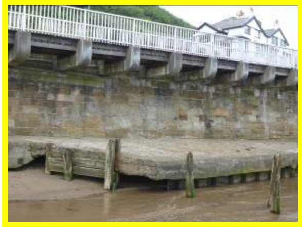
Voiding and undermining of concrete apron (\D0702C04)
