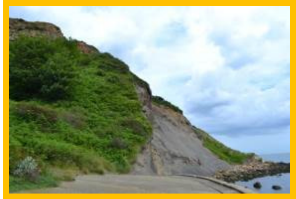
Debris fan at south end of MU6/8. (Partly Active in June 2016)
