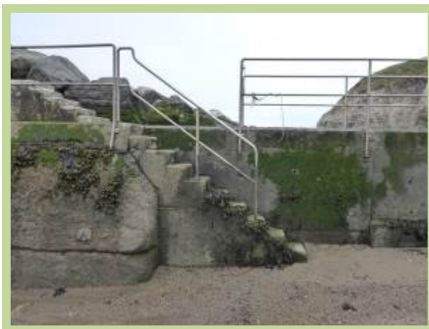
Local abrasion, cracking and spalling, but otherwise good condition (/0403C03)
