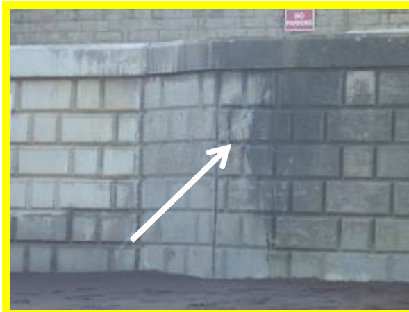
Vertical cracks in wall protecting recent development (/1201C06)
