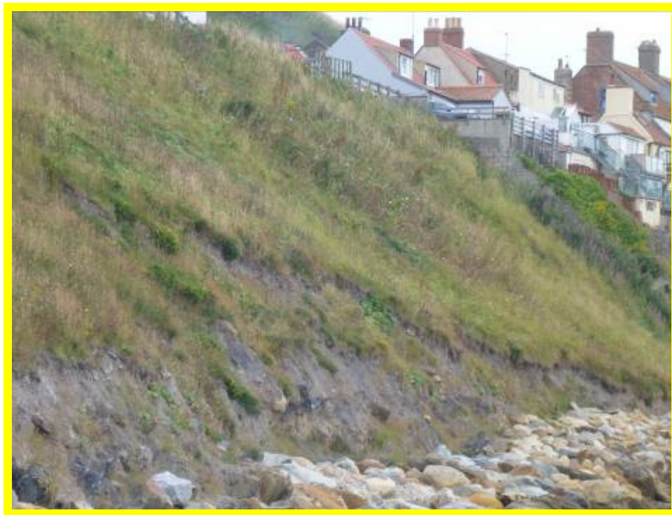
MU12/1 Slumps in lower cliff (Locally Active)
