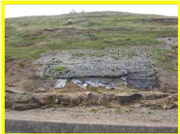
MU11/1 Exposed previous repairs (Locally Active)
