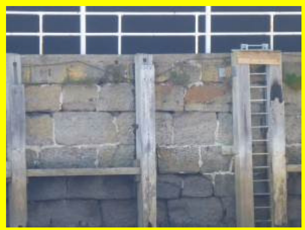
Some open and some sealed joints in pier wall near lighthouse (/1301C03)
