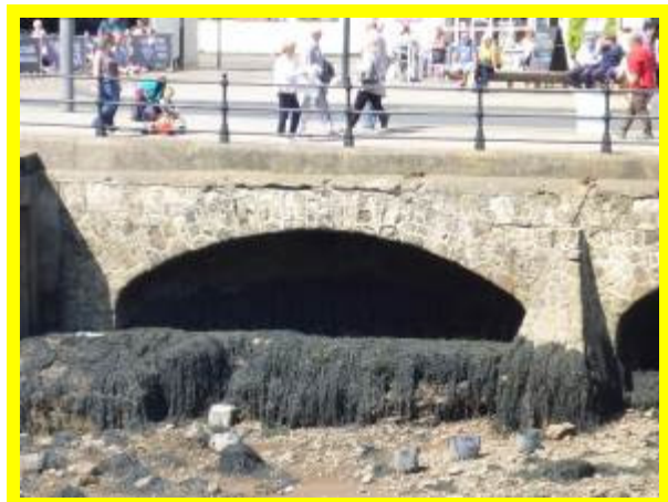
Some open and some sealed joints in pier wall near lighthouse (/1301C05)
