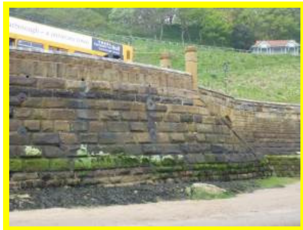
Masonry sea wall at The Spaw access steps in fair overall condition (/1301C27)
