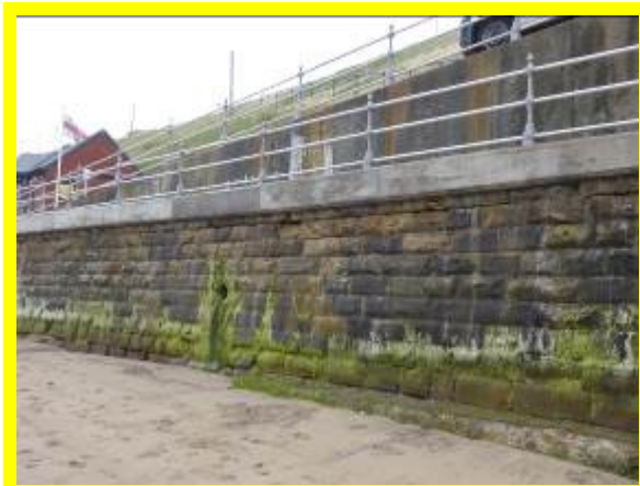
Fair condition masonry wall with recent capping beam to repair previous defects (D0802C07)
