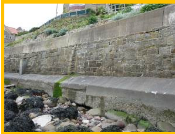
Undermining, cracking and open joints in sea wall (/0601C03)
