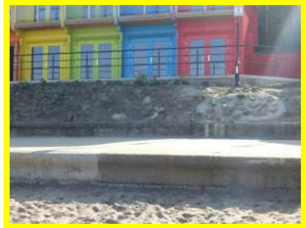
Previous repairs to stone revetment at rear of promenade (/1201C05)
