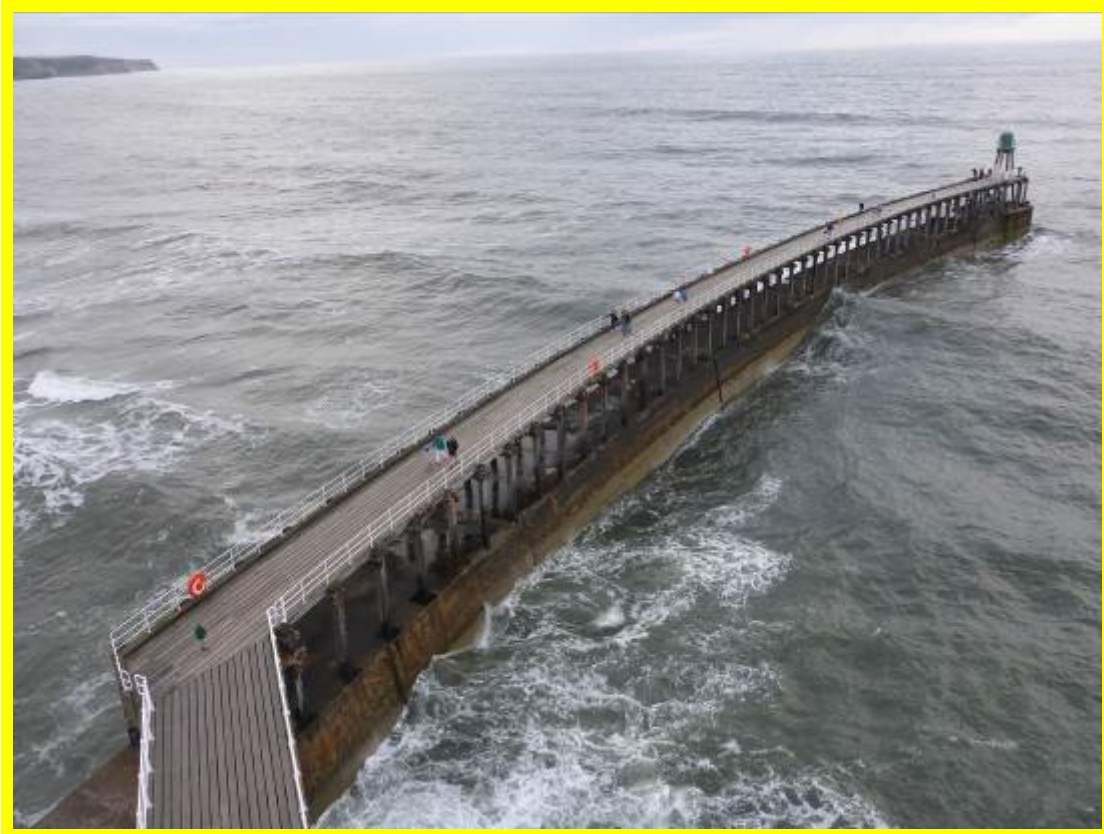
West Pier extension, generally in fair condition (\803C01)
