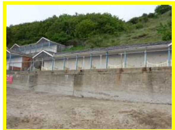
Longitudinal cracks in rear wall (/1602C01)
