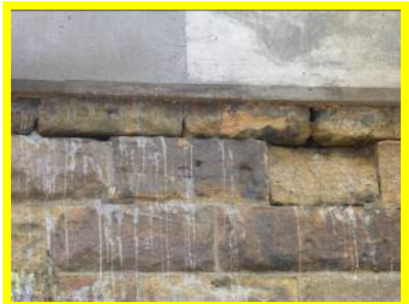
Local defect (sunken blockwork) below new capping beam (D0802C07)
