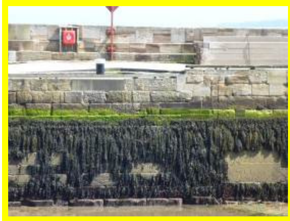
Previous repairs to inner-facing wall of East Harbour outer pier (/1301C16)
