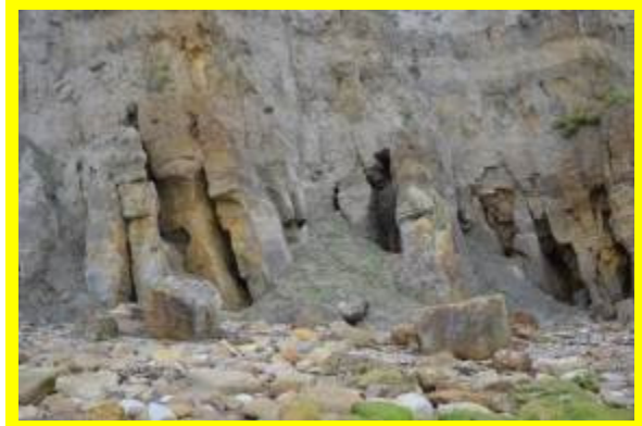
Local rock fall and debris cone in MU24/P (Locally Active in June 2016)
