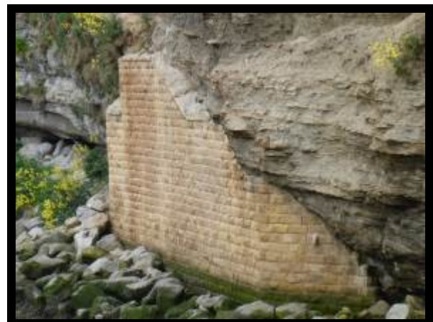
Works completed upstream of bridge in 2013 to repair collapsed cliff (no asset ref)
