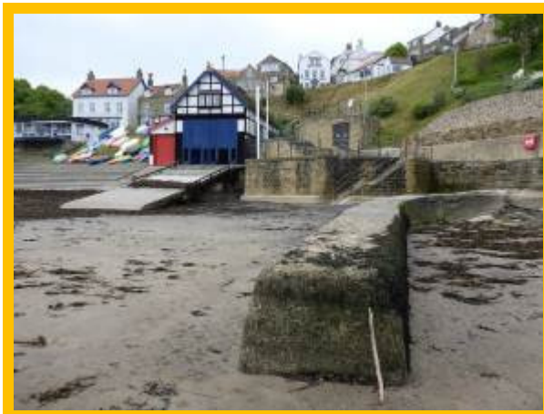
Undermining, cracking and open joints in sea wall (/0601C02)
