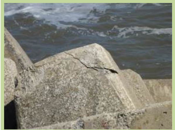
Locally cracked Accropode unit but otherwise good condition revetment (/1202C04)
