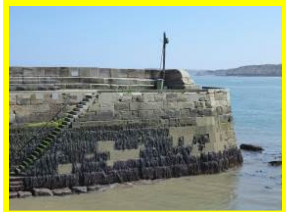
Previous repairs to inner-facing wall of East Harbour outer pier (/1301C16)
