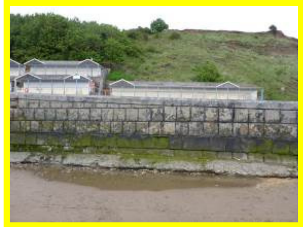
Abrasion of concrete toe apron (/1602C09)
