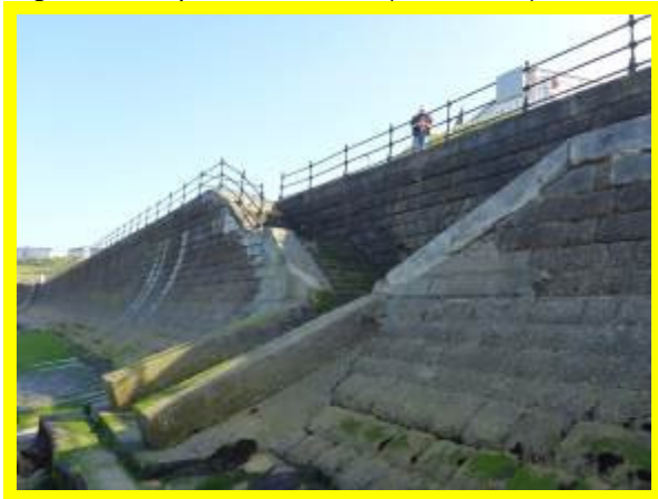
Previous repairs to wing-wall (/1201C07)
