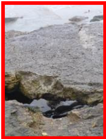
Large hole in deck surface with visibility through to foreshore due to size of void underneath (/1402C04)
