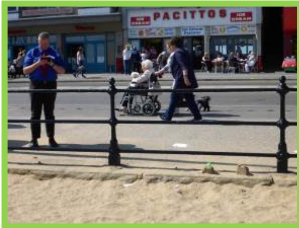
Beach levels flush with promenade at north end of Foreshore Road seawall (/1301C15)
