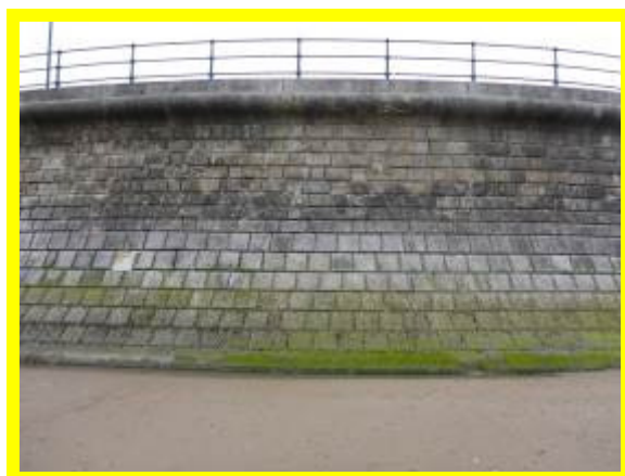
Royal Parade sea wall in fair condition but with some blockwork abrasion (/1602C04)
