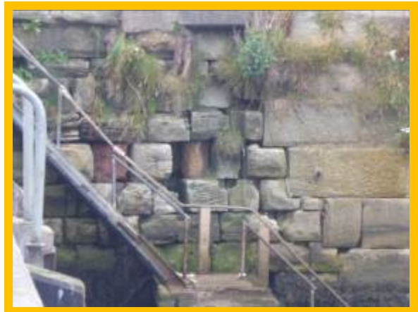
Local poor condition of quay wall due to open joints between blocks (\803C06)
