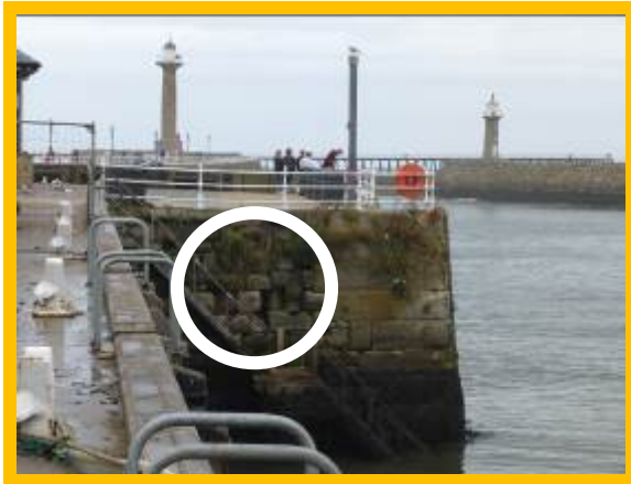
Local poor condition of quay wall due to open joints between blocks (\803C06)
