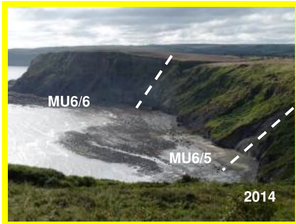
MU6/5 – The unit was substantially vegetated in 2014 but active marine erosion and localised failures in the cliff are evident (Locally Active).
