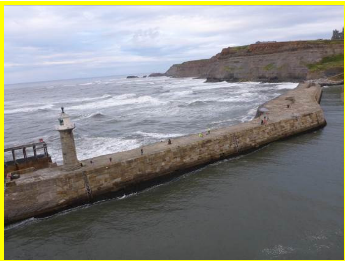
East Pier, generally in fair condition but locally very poor (803C03)
