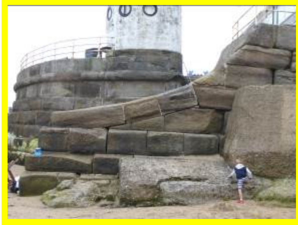
Open joints in wing wall to access steps (\D0802C12)
