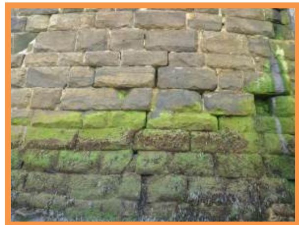
Typical defects on blockwork wall (/1003C04)
