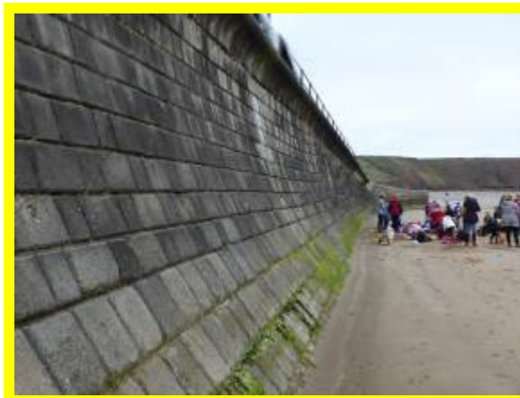
Sea wall near Ravine Road in fair condition (/1602C06)
