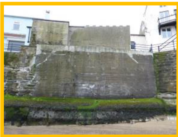
Cracking, open joints and vegetation growth (/0402C22)
