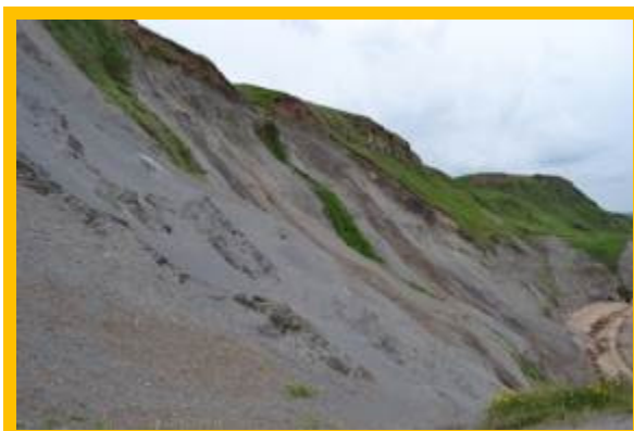
Steep cliff with debris flows. MU8/3 Partly Active in June 2016
