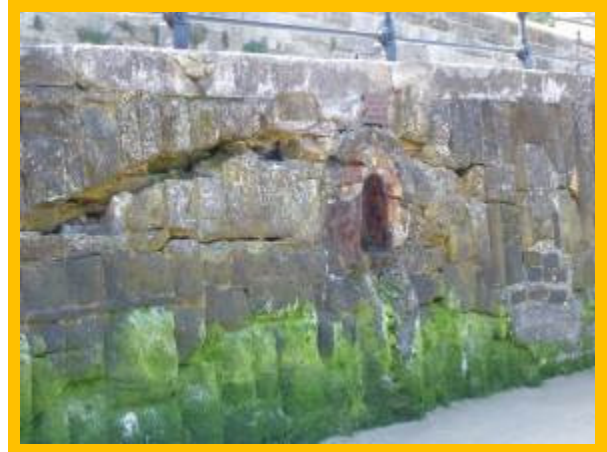
Vertical crack in wall above access ramp (/1301C10)
