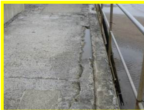
Abrasion on lower deck of North Breakwater (/0402C01)
