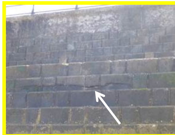
Longitudinal crack in blockwall wall (/1201C08)
