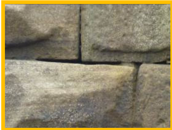
Local poor condition of West Pier due to open joints between blocks (\803C02)
