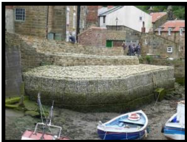
Works completed upstream of bridge in 2013 to repair collapsed wall (no asset ref)
