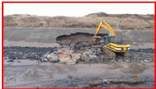
Previous temporary repairs to sloping revetment at Sandsend Road (\D0702C02)
