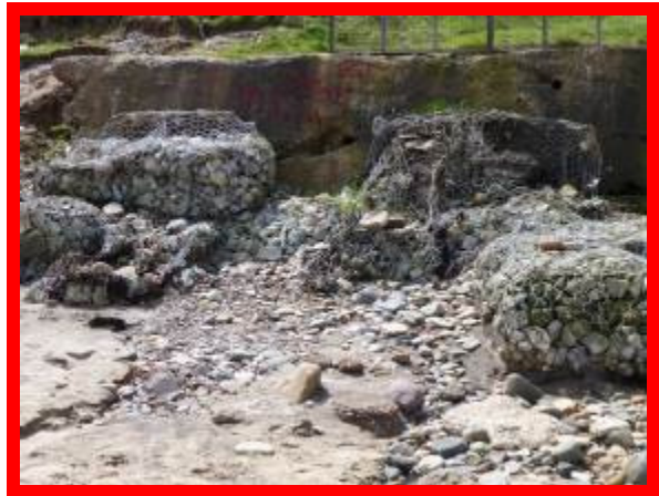
Failed gabion baskets at surf shop car park beach access (no asset reference)
