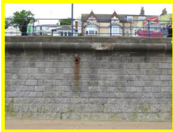
Sea wall south of Ravine Road in fair condition but with damaged coping and lower blockwork abrasion (/1602C08)
