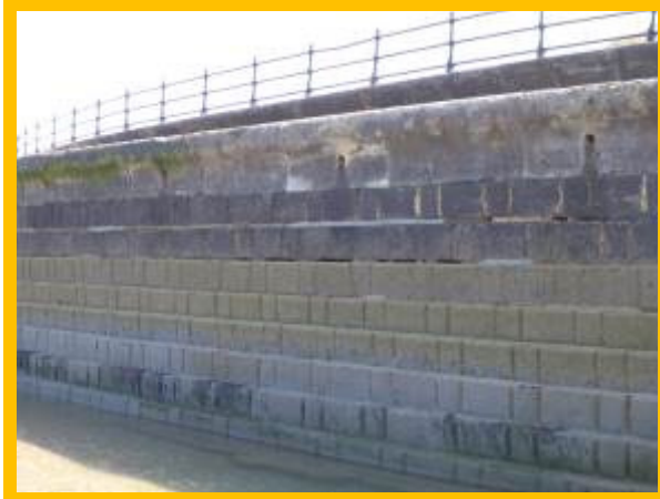
Concrete block wall with open joints and heavy abrasion (/1303C02)
