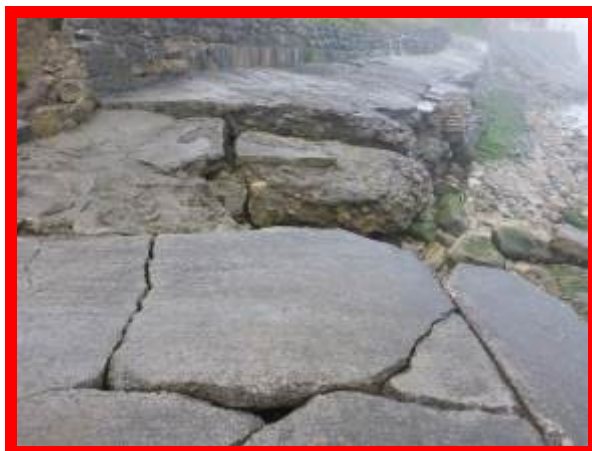
Cracked concrete at landing at beach access (/1402C06)
