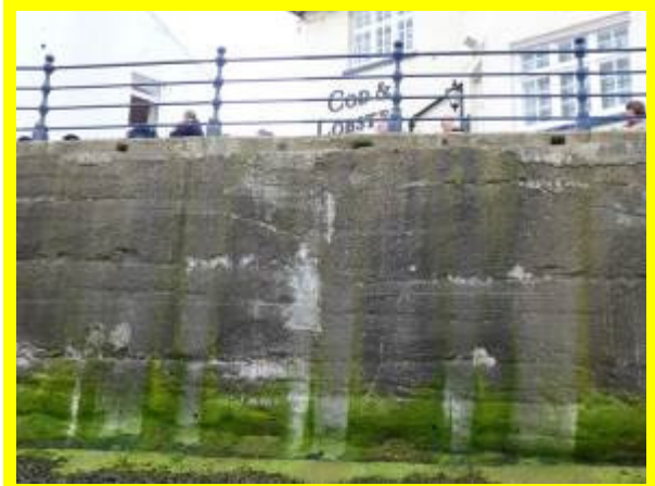
Abrasion and cracking to seawall face and crest (/0403C05)
