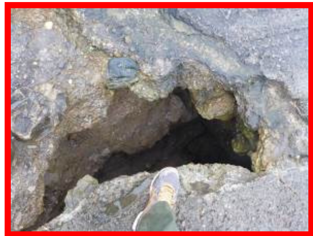
Large hole in deck surface (/1402C04)
