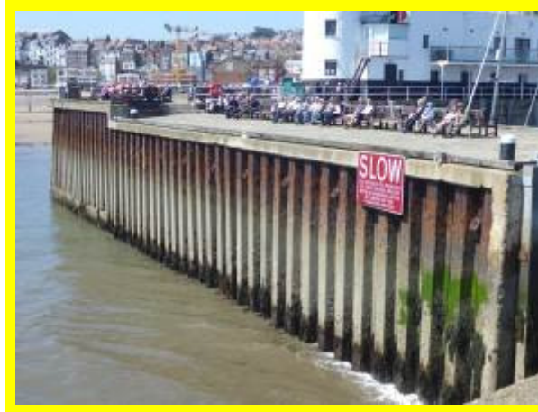
Corroded steel sheet piling (/1301C17)
