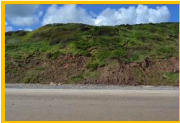
Till cliffs beneath Reighton Sands Holiday Village. MU27/BR Partly Active in June 2016
