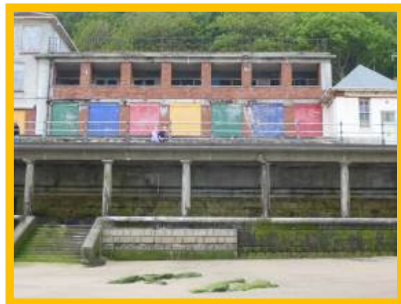
Previous repairs (Dec 2013) at the open colonnade remain effective, but extensive open joints remain in lower wall (/1302C01)
