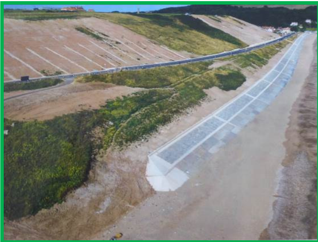
Oblique view of coastal defences at Sandsend Road in 'as built' condition showing subtle 'S' curve (\D0702C02)
