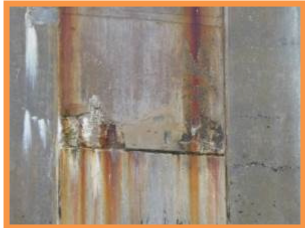
Typical defects on large sea wall (/1003C02)
