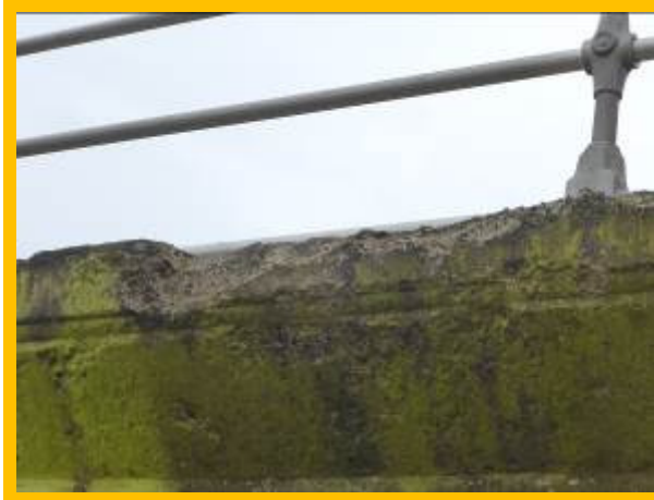
Damage to sea wall coping (D0802C03)
