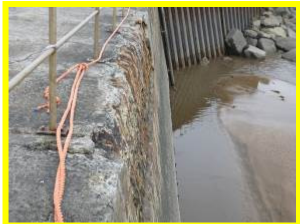
Abrasion and rust-staining on inner-facing edge of North Breakwater (/0402C01)
