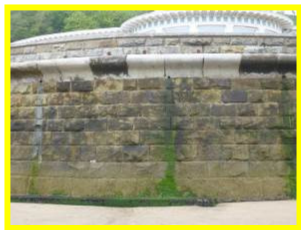
Previous repairs to wave deflector wall in front of the Sun Court (/1301C28)
