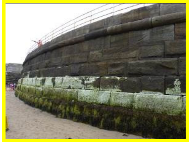
Battery Wall, with some open joints between blocks (\D0802C12)
