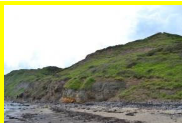
Steep mudstone cliffs with overlying shallower sloping till with local slumps. MU7/4 Locally Active in June 2016
