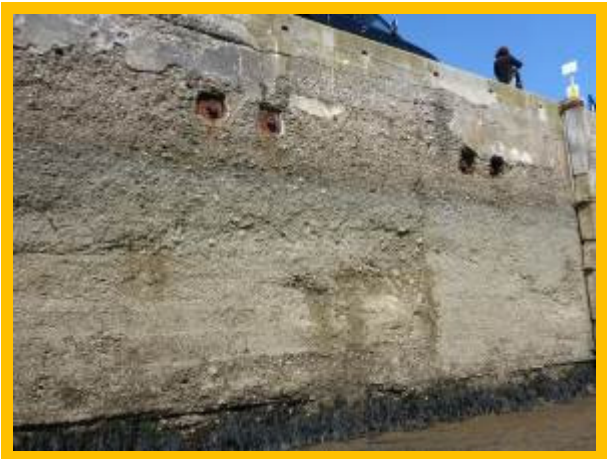
Spalling and loss of render in south face of West Pier wall (/1301C07)
