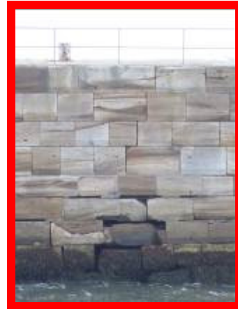
Local very poor condition of East Pier due to open joints and settled blocks (\803C04)
