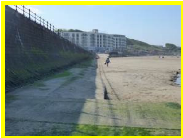
Toe apron with algae growth (/1201C07)
