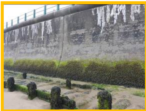
Poor condition sea wall (D0702C01)
