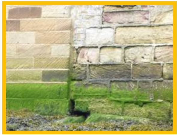
Gap at base of interface between new and older walls in front of RNLI station (/0402C06)
