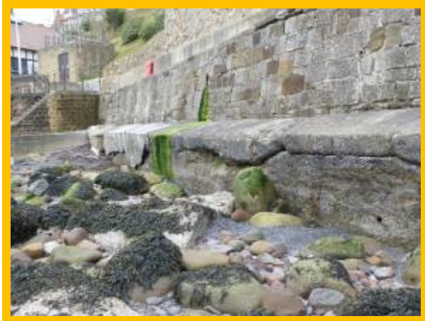
Previous repairs to toe apron next to heavily abraded section (/0601C03)
