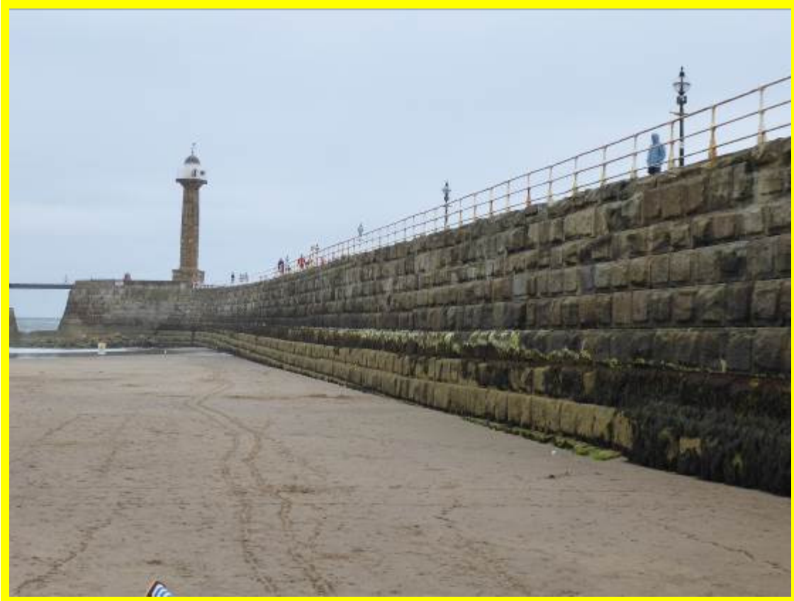
West Pier, generally in fair condition but locally poor (803C02)
