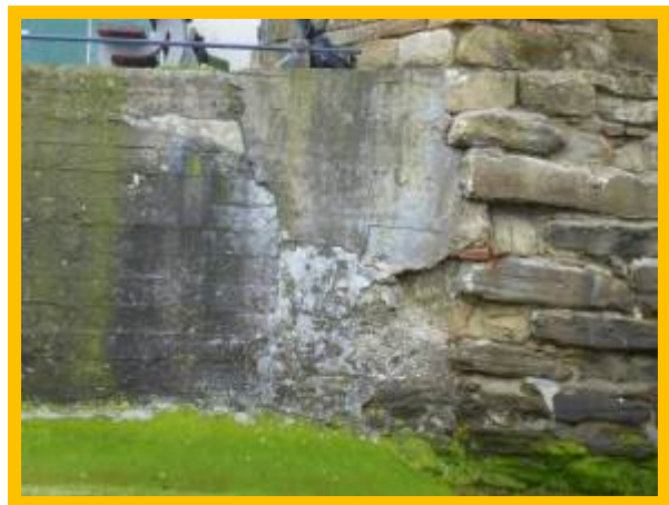
Cracking, open joints and vegetation growth (/0402C22)
