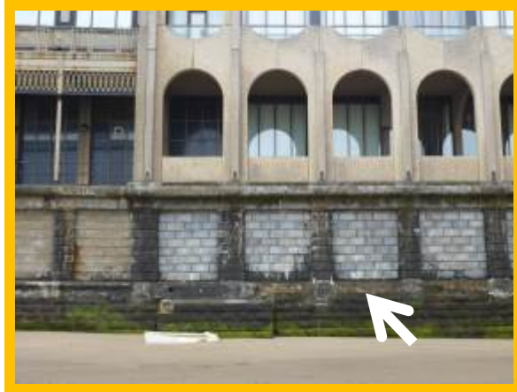
Spalling to the lower splash beam at closed colonnade section (/1301C29)
