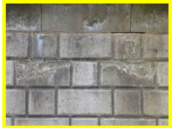
Abrasion damage and open joint in sea wall south of Cargate Hill (/1602C03)
