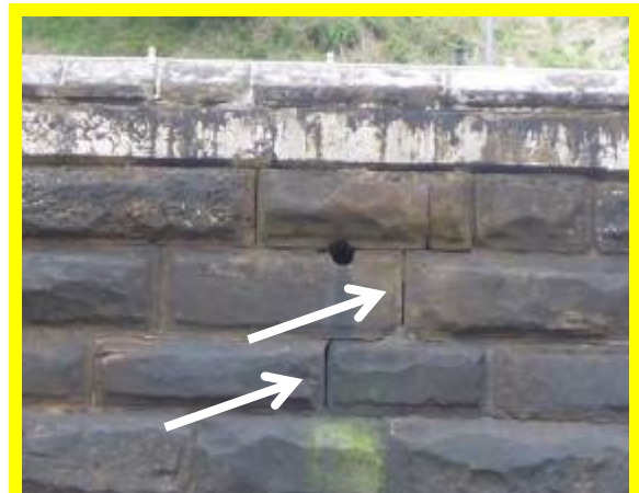
Example of gaps between blocks in sea wall (/1301C27)
