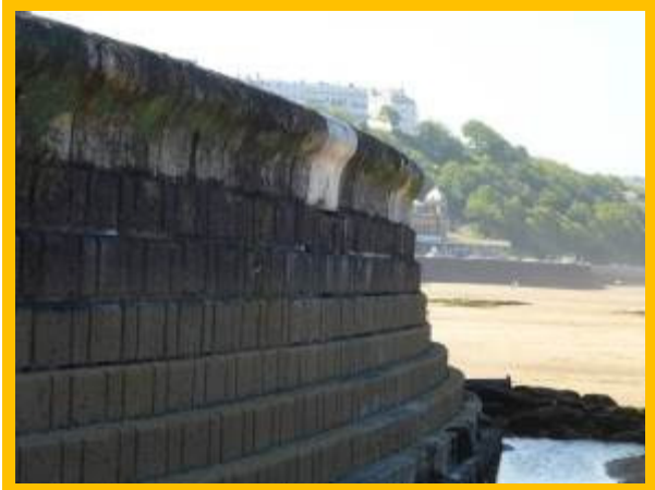
Previous repairs to wave return coping (/1303C02)
