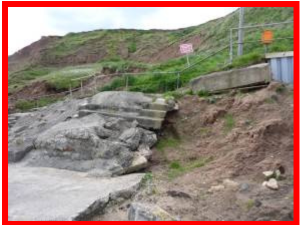
Slumping cliffs adjacent to steps leading to outflanking – northern end (/1402C04)
